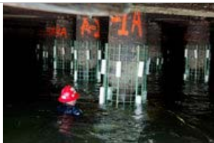
Ángel Franco/The New York Times Workers fit steel cages and fiberglass molds around each piling then pump in concrete.
