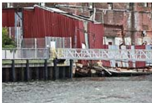
Fred R. Conrad/The New York Times A new bulkhead at the Schaefer Landing ferry terminal in Williamsburg, Brooklyn, abuts a collapsing wharf built on wooden piers.
